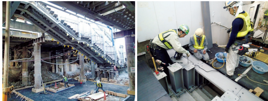
仮設階段施工状況。既存階段の撤去の様子(左)と踏面プレート設置の様子(右) Temporary stairway construction: removal of the existing stairway (left) and kick plate installation (right)
